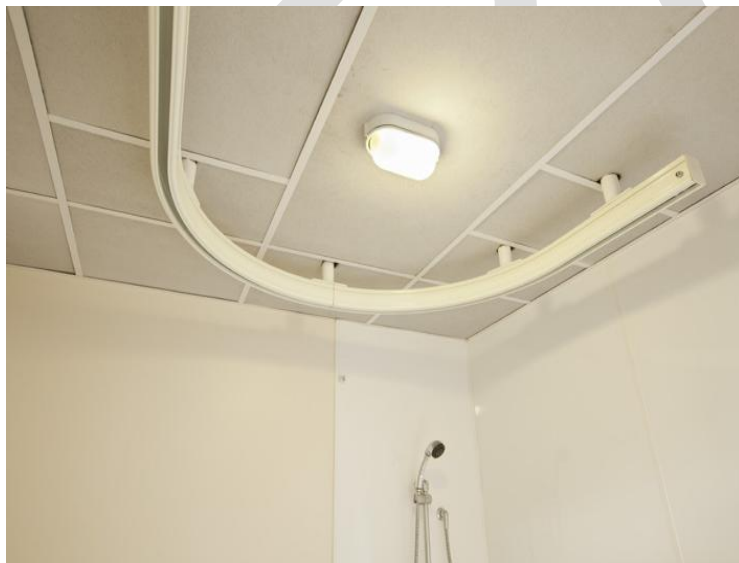
Figure 3.5.2 – Curved Ceiling Tracking in Bathroom
